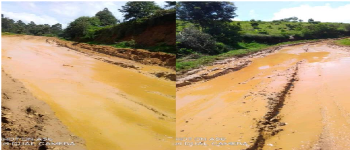
Photo 1 and 2: Poor state of roads in the rainy season in upper wabane
